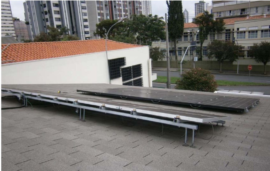
Figure 4. Green office photovoltaic system. Source: [13]
