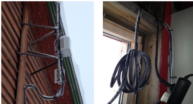
Figure 5. Icing on external power cable
